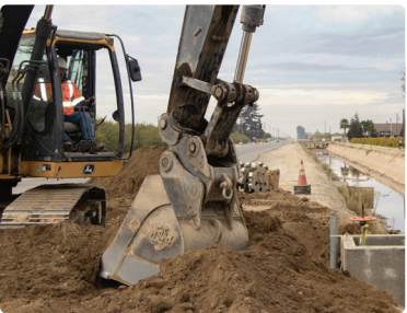
Construction crews add a turnout that allows water to flow from FID's Herndon Canal to Biola CSD's existing storm drain basin.
