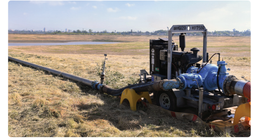
Temporary pumps for flood diversion and recharge from the California Department of Water Resources (DWR).
