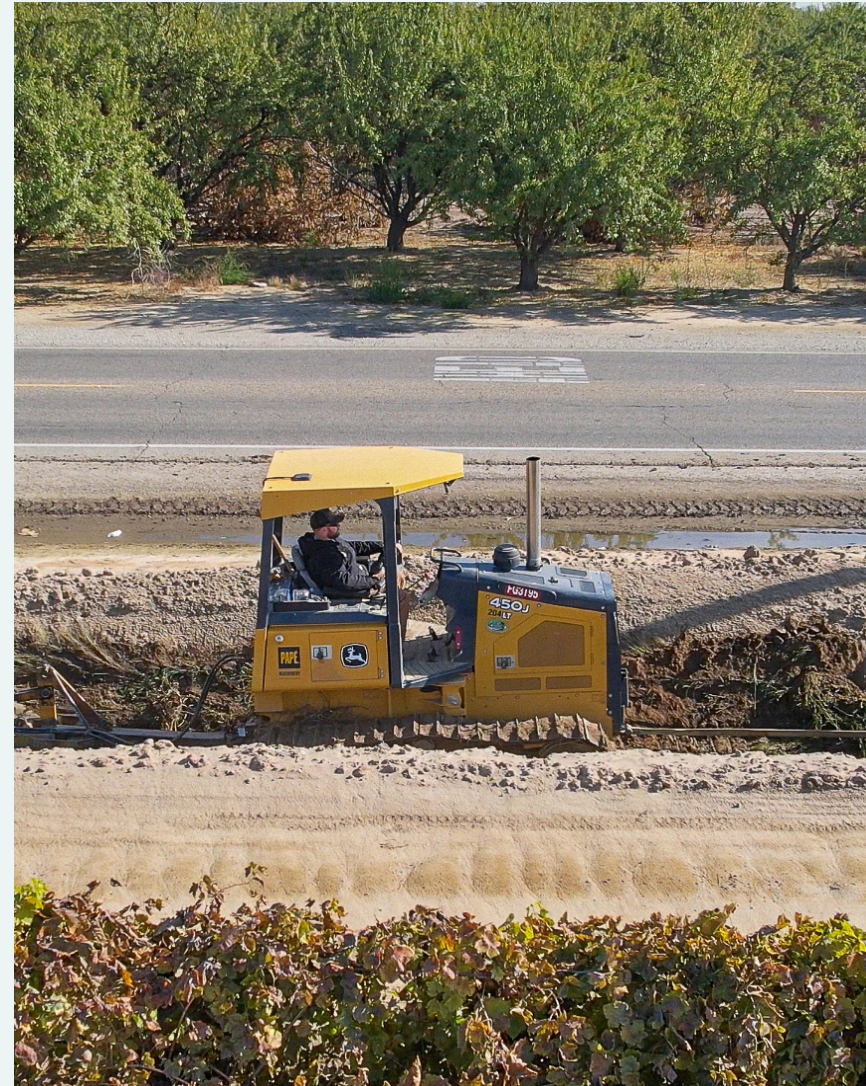
A sloping crew removes weeds and silt from the open channel by pulling a sloping machine through the channel's interior. This work allows for more efficient delivery of water to growers as well as better ground-water percolation along the channel itself.
