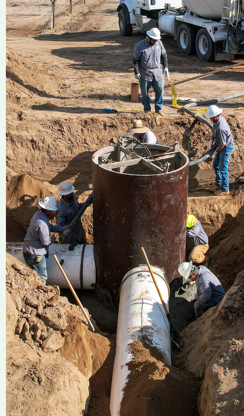
An FID construction team prepares to pour concrete for a structure along the Minor Thornton Canal.
