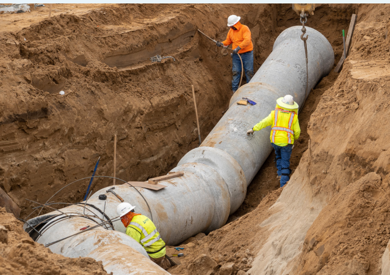
FID-contracted workers inter-tie the Savory Groundwater Recharge Basin to the Oleander No. 16 canal with RGRCP Pipeline.
